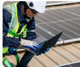
Solar PV Installation for Suppliers
