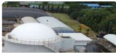
Process sludge through digester system
