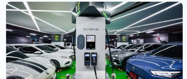
130 stations installed EV charging system to encourage clean electrical energy
