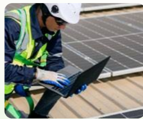
Solar PV Installation for Suppliers
